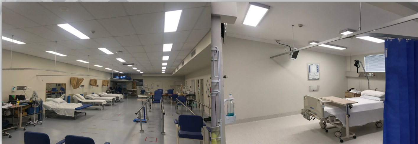
Corona™ Panels installed throughout the Hospital.
